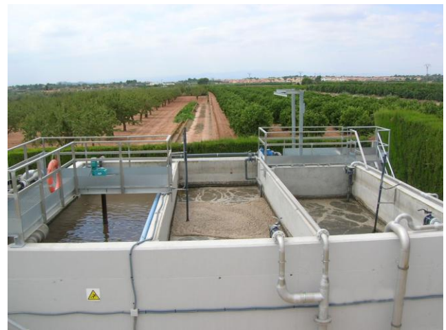
Figure 3: Plant after upgrade
