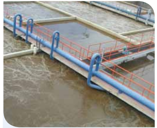
Municipal, Upgrade – Mexico (58,300 m 3 /d)
