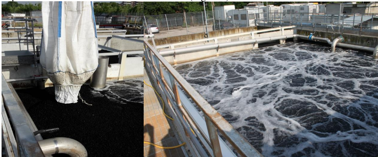
Figure 6. Introduction of Aqwise biomass carriers (left) and carriers mixing in the aerobic stage (right)
