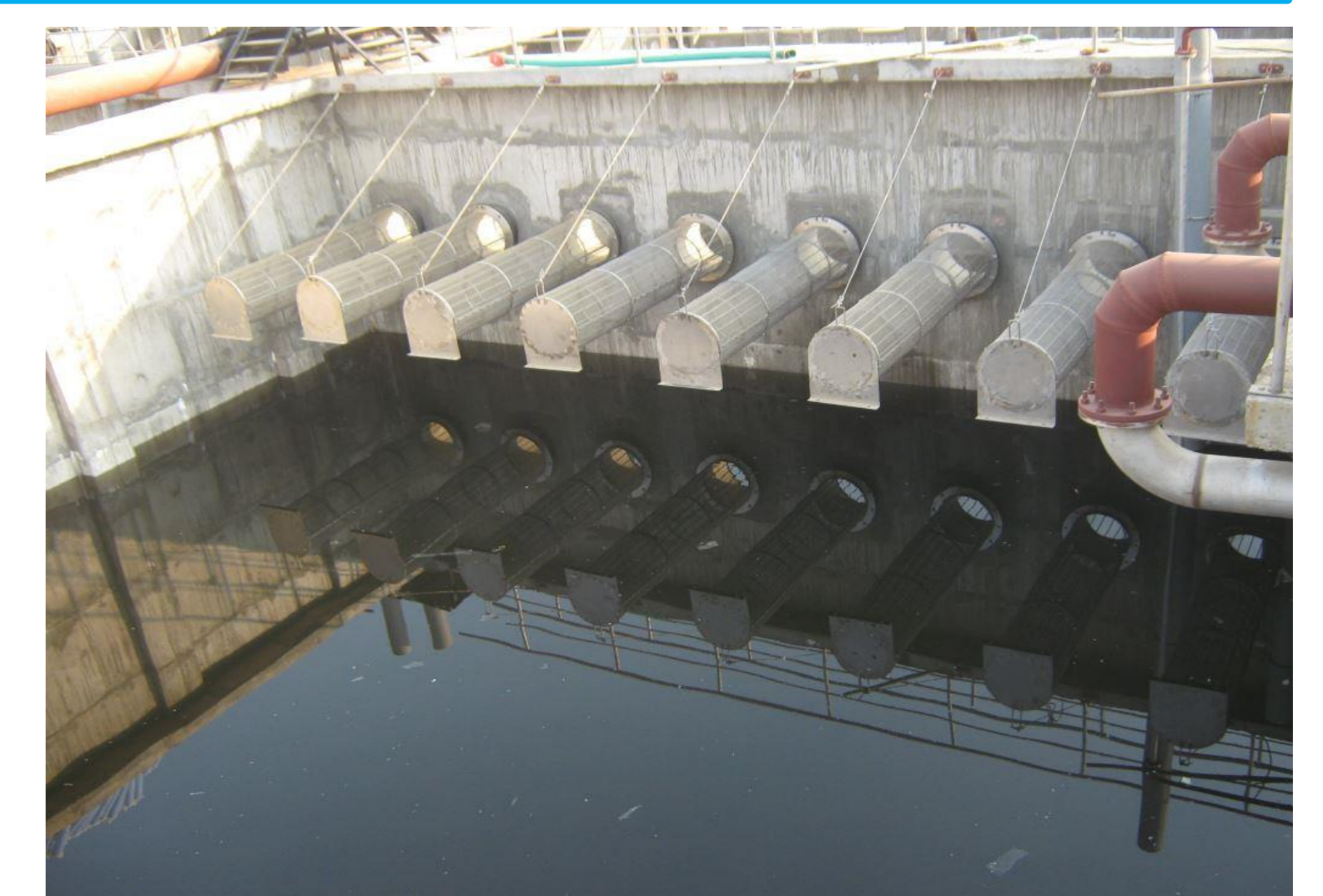
Figure 5 – Retention screens in aerobic stage
